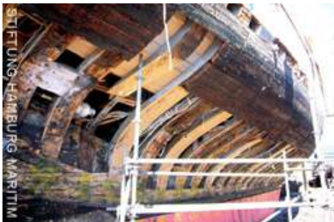
New oak frames were installed after the removal of Artemis' infected planking.
